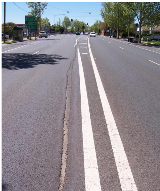
Figure 1. Slippage of butt joint in fabric used as a SAMI under ultra thin asphalt surfacing
