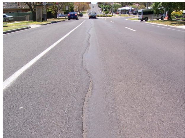
Figure 2 Slippage of butt jointed fabric in SAM seal
